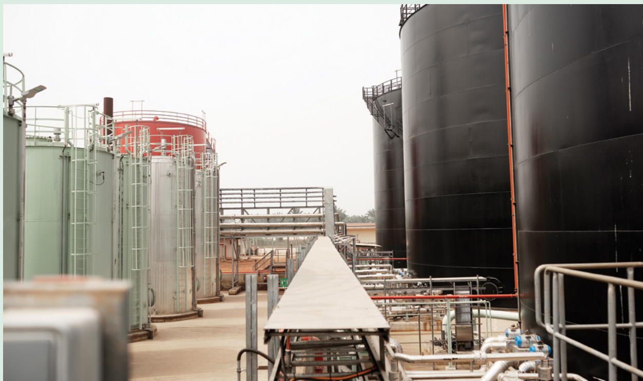
A 120MW Thermal Power Station in Maria Gléta, Benin
